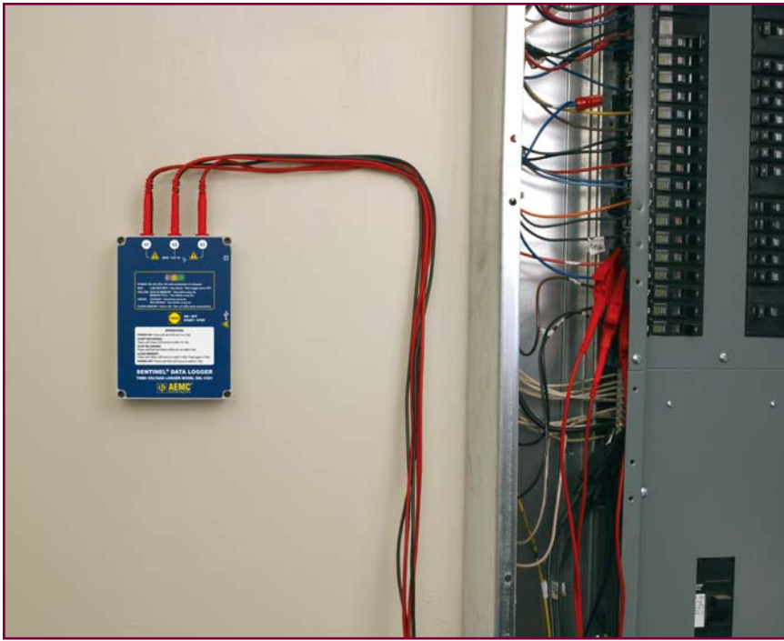
Model SDL V301 recording three-phase voltage on a lighting panel.
