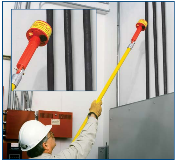
Model 275HVD checking for live voltage on main feeder
